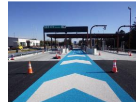
KEN-O EXPWY Tochigi Colored pavement in the ETC lane at the Bando Interchange.
